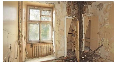
Room of the restituted hospital in disrepair
